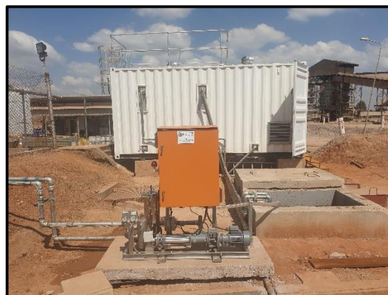
Figure 2: Outside view of the containerized Hydraspin and SRS system on the outside.
