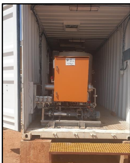
Figure 1: Hydraspin system inside the container.
