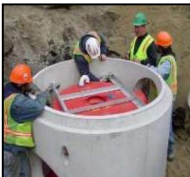
Figure 2: Downstream Defender installation
